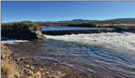
The Weir across the Liawenee Canal and the run up to the fish trap on the left
