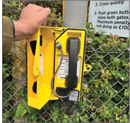
The Boom-gate connection
